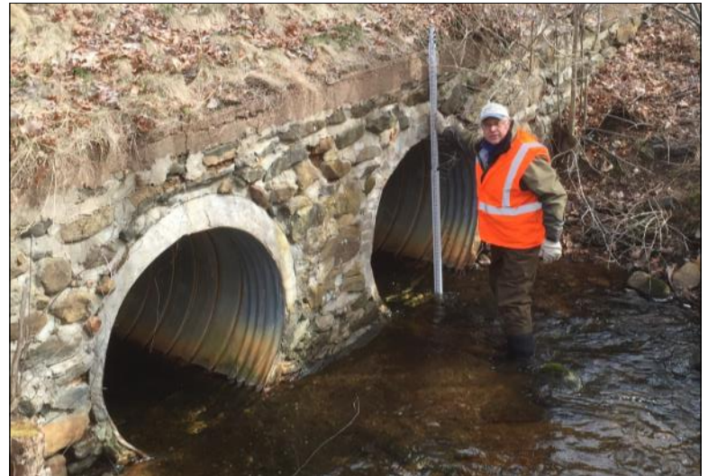
Mianus TU President Tony Hill, measures culverts during a training on assessing barriers to fish passage in streams with the state of Connecticut fisheries biologists.
